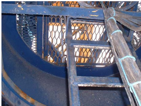
Figure 2 – Cables Attached to Ladder
