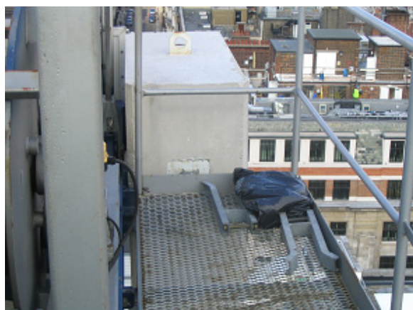
Figure 2 – Poorly Stored Components
