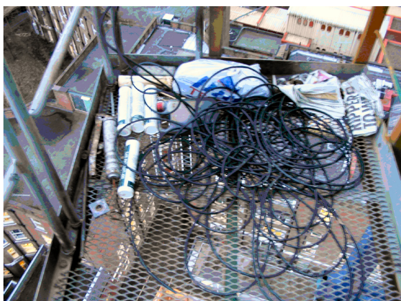
Figure 1 – General Loose Material
